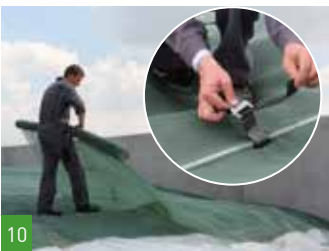
10 Pull the plastic and then the tarpaulins over the pit. Connect all the tension straps with the buckles and pull the tarpaulins together.
