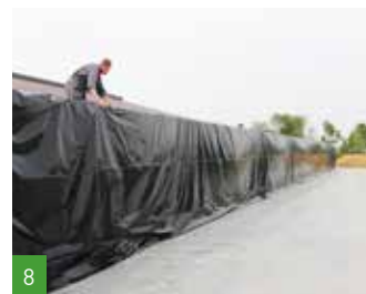
8 Lay the plastic over the walls (see over). Provide 10-20 cm clearance on the floor.
