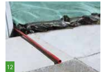
12 Connect the 2 red PVC pipes to the grey PVC pipes at the pit entrance as marking and for rainwater drainage.
